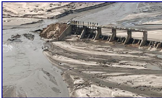
Aerial view of what's left of the Spencer Dam on the Niobrara River in Nebraska, which gave out March 14, 2019. (Photo: State of Nebraska)
