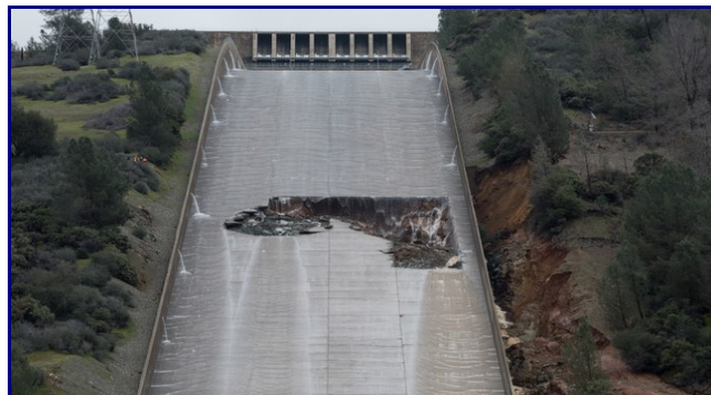
The Oroville Dam Spillway-- the damage
