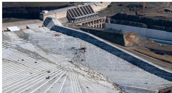
An aerial overview of the finished roller-compacted concrete splashpad, while work continues on the concrete cap (upper left) below the Lake Oroville emergency spillway weir at the Butte County, California site. Photo taken January 24, 2019. Kelly M. Grow / California Department of Water Resources, FOR EDITORIAL USE ONLY
