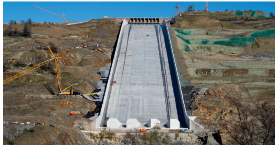
Cleanup work continues surrounding the newly completed Lake Oroville main spillway in Butte County, California. Photo taken January 22, 2019. Kelly M. Grow / California Department of Water Resources.
