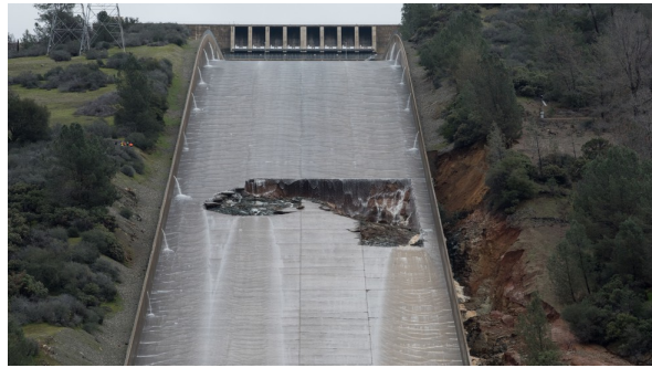
The California Department of Water Resources suspended flows from the Lake Oroville flood control spillway after a concrete section eroded on the middle section of the spillway. Photo taken February 7, 2017. Kelly M. Grow/ California Department of WaterResources
