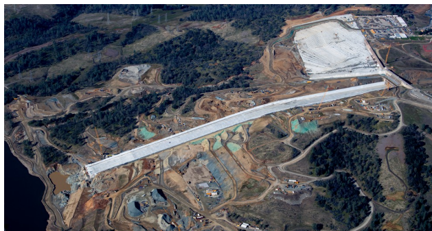
An aerial overview of the recently completed Lake Oroville main spillway during Phase 2 of the recovery efforts. Work continues on the concrete cap below the Lake Oroville emergency spillway weir at the Butte County, California site. Photo taken January 24, 2019. Kelly M. Grow / California Department of Water Resources, FOR EDITORIAL USE ONLY
