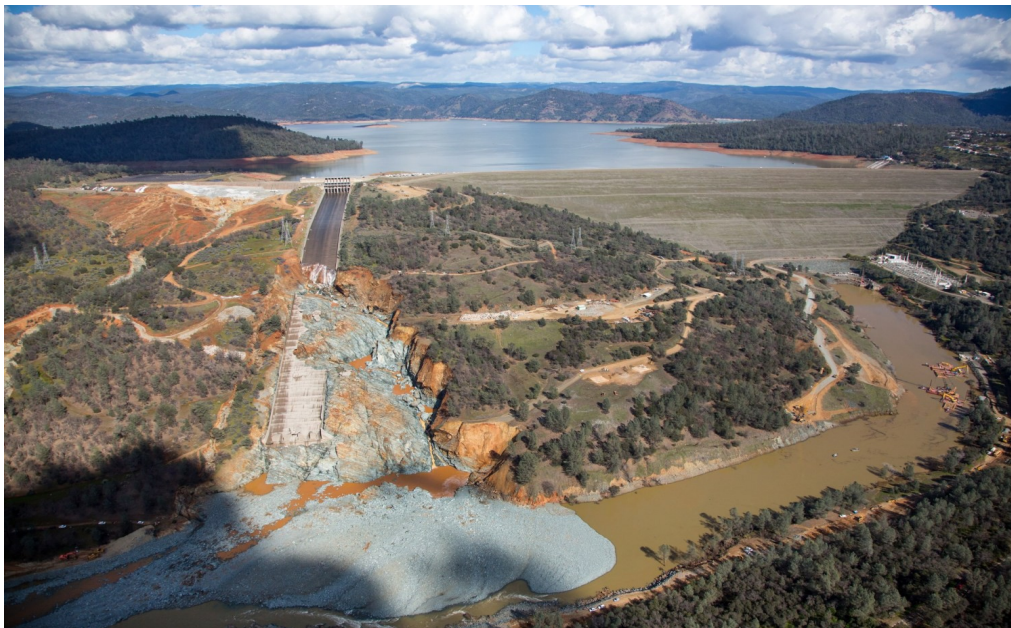
An aerial view of the damaged Oroville Dam spillway and the huge debris field below it, in a photo taken on February 27, 2017. Photo courtesy of Dale Kolke / California Department of Water Resources
