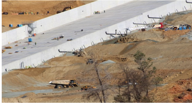
Crews Tuesday work on backfilling the side walls of the main Oroville Dam spillway.
