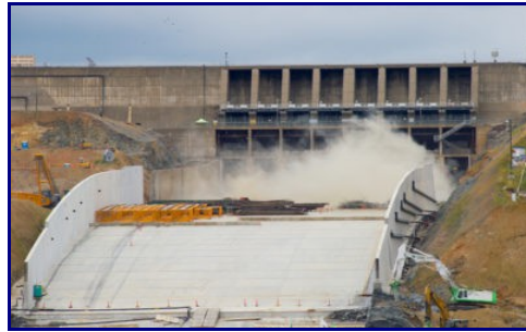
A controlled blast breaks up a section of the original upper chute of the Lake Oroville main spillway in Butte County, California. Photo taken May 16, 2018. Kelly M. Grow/ California Department of Water Resources, FOR EDITORIAL USE ONLY
