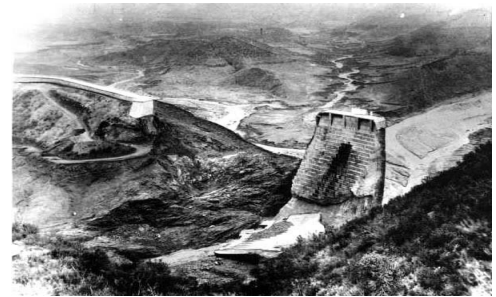
View of the St. Francis Dam just hours after its catastrophic failure (11:57 p.m., March 12, 1928).
