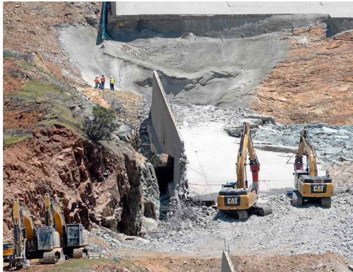
Heavy equipment works Wednesday to break up remaining concrete on the lower part of the damaged main Oroville Dam spillway so a replacement can be constructed. (Bill Husa — Mercury-Register)
