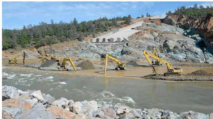
Excavators remove debris from the Diversion Pool below the main Oroville Dam spillway in this photo from March 29. (Bill Husa-- Mercury-Register)
