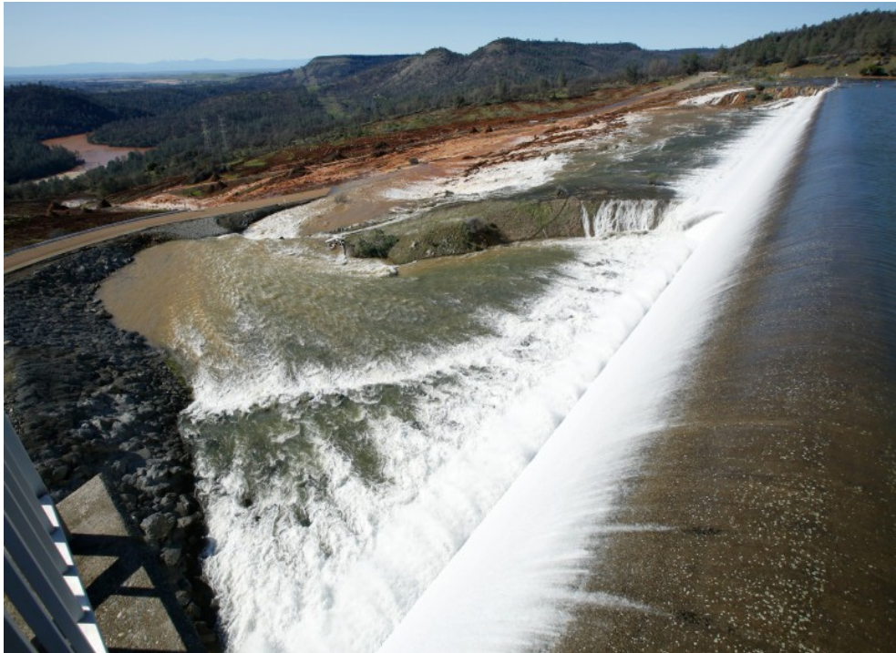
Water flows over the emergency spillway, eroding the supporting soil.
